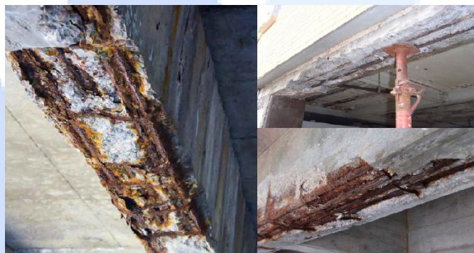
Figure 5. Corrosion in the middle lower part of the concrete beam
