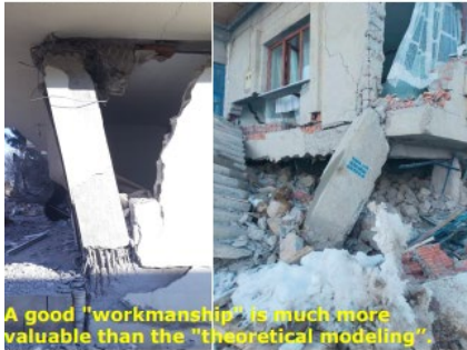
Inadequate steel reinforcement (in size and number of longitudinal bars)
