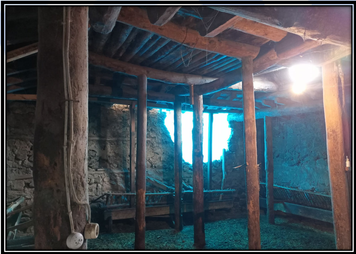
Figure 13. An example of the damage observed after the April 13, 2023 Aziziye Earthquakes
