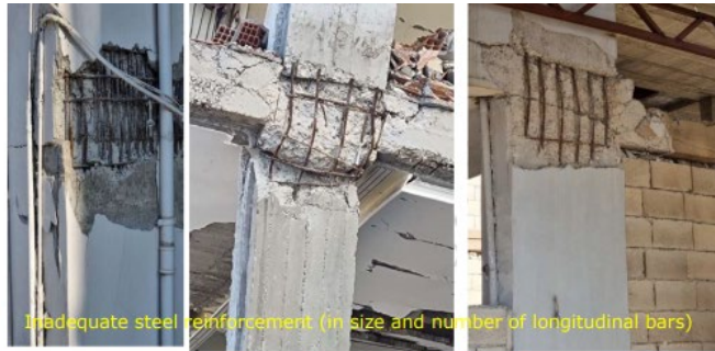
Lack of column confinement and poor detailing
