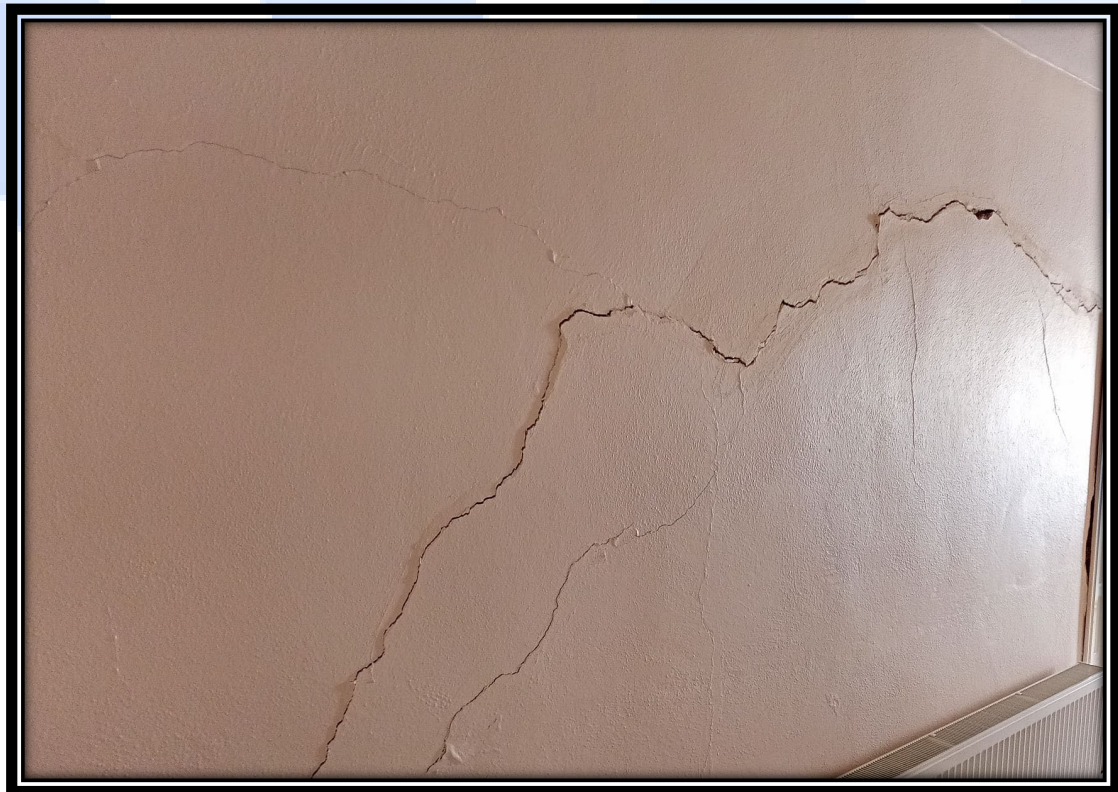
Figure 11. An example of the damage observed after the April 13, 2023 Aziziye Earthquakes
