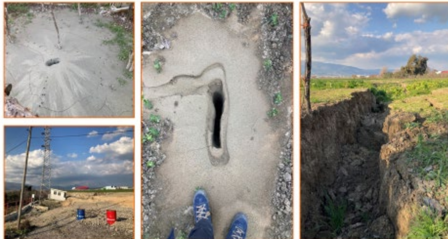
Earthquake-triggered liquefaction phenomena and subsidence reported from the northeastern end of the Hatay city center. Source: https://twitter.com/geodesist_a/status/1624410147853414400
