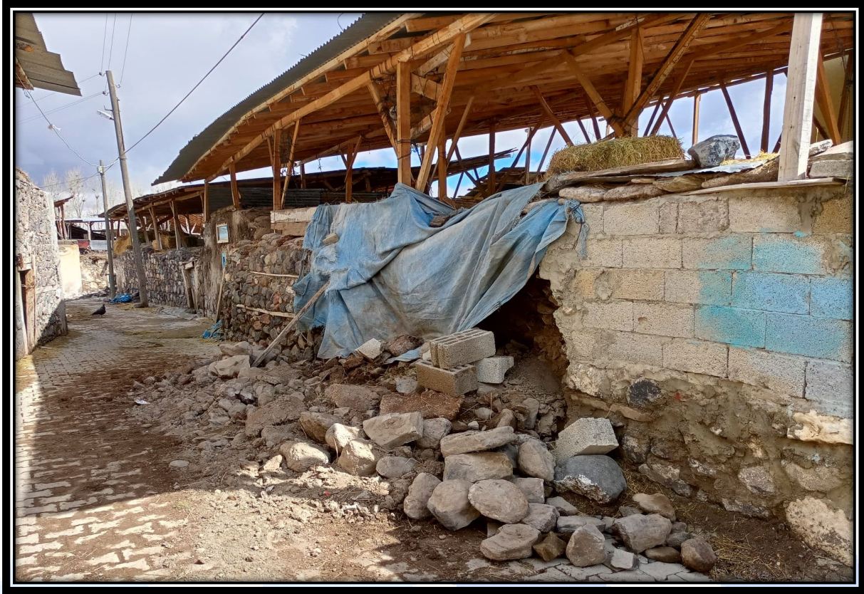
Figure 14. An example of the damage observed after the April 13, 2023 Aziziye Earthquakes
