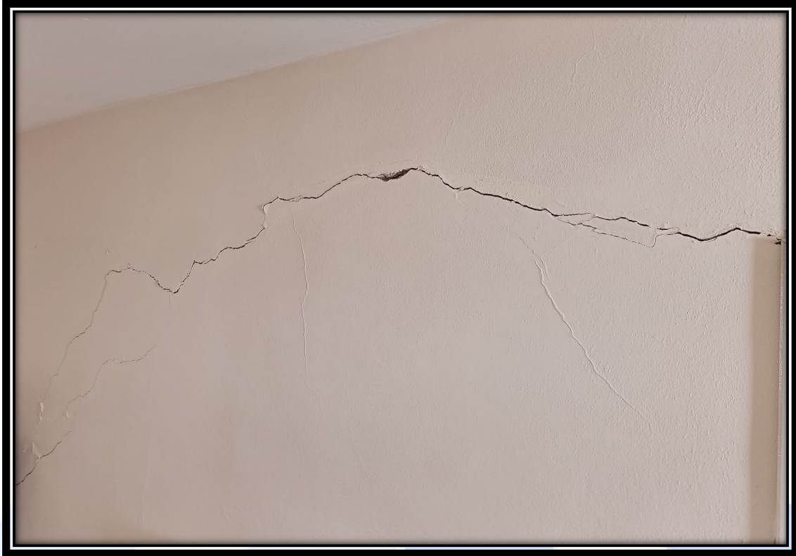
Figure 12. An example of the damage observed after the April 13, 2023 Aziziye Earthquakes
