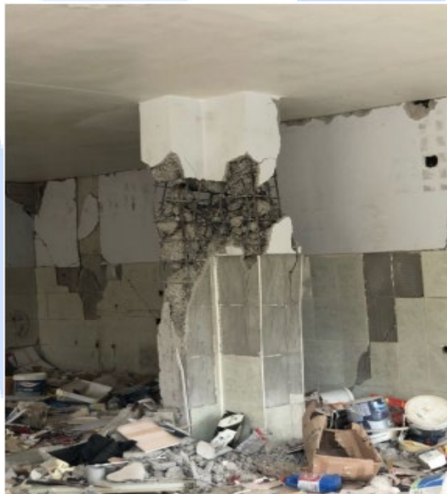
L-shaped central column failure from the ground story of a framed building.
